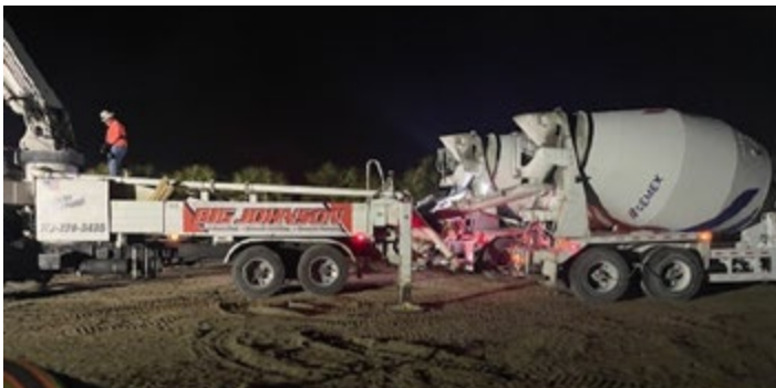
27 Cement Trucks start pouring at 0200 on 05 May to complete the slab in 10 hours.
