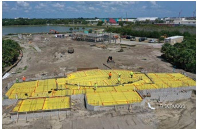
The Amphitheater in early May ready to put the cement slab. Not great progress on the concessions building to the West.
