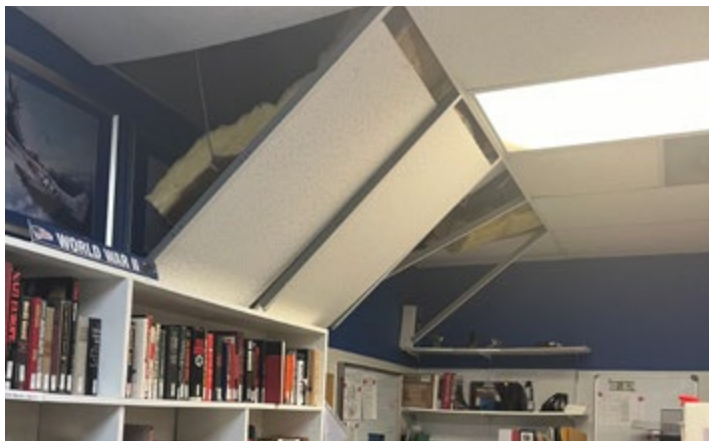
Hurricane Milton loosened the Library ceiling tiles but it was an easy repair
